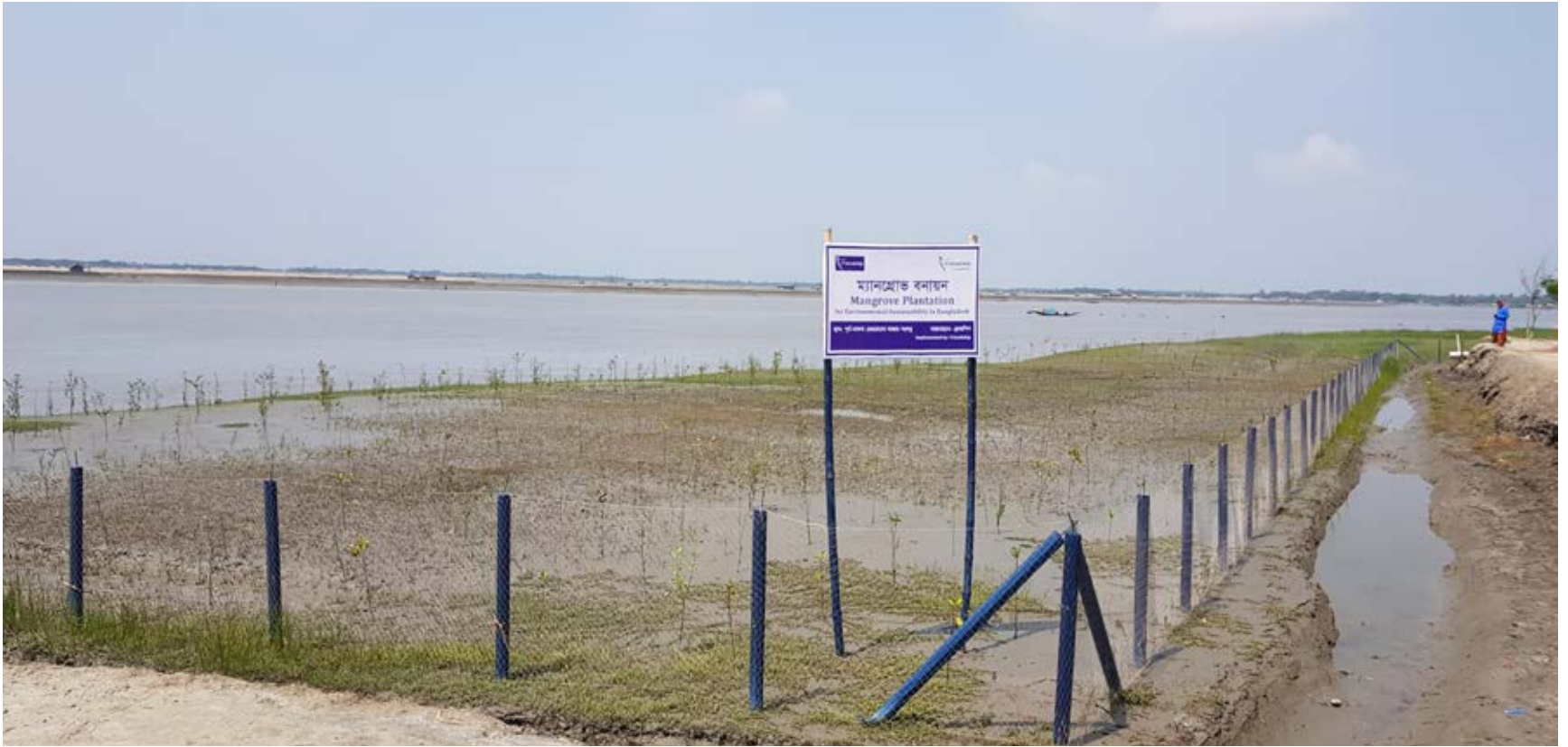
The mangroves are being planted in the flatlands just outside the embankment to offer protection against the waves.
